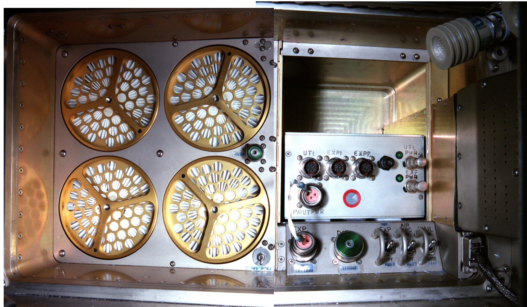
Figure MG-281 Interior of MGBX
